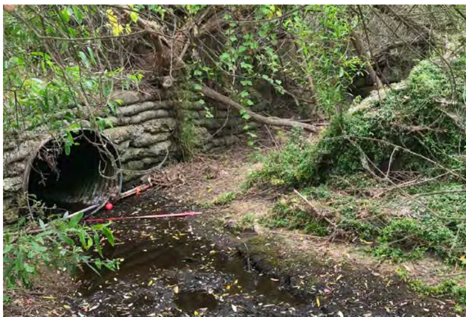
Photo 1. Photograph dated 5/31/2018, taken by Anita M. Hayworth of DUDEK, showing the makeshift headwall, consisting of stacked burlap sacks of concrete. This unpermitted structure would not be replaced as part of the Quail Meadows project. Also shown is the upper end of the failed 48-inch corrugated metal pipe that would be sliplined as part of the project.
